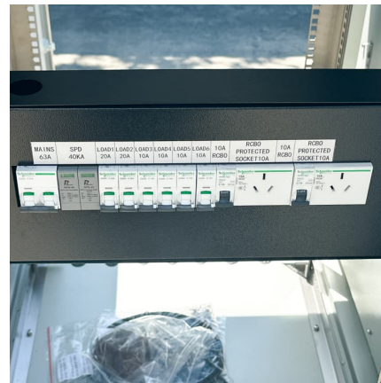
port of spain containerized energy storage system
