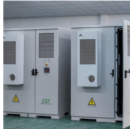
(a) Image of one supercapacitor energy storage
