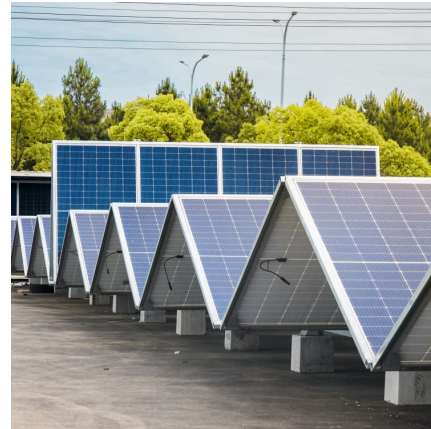
Utility-Scale PV , Electricity , 2023 , ATB , NREL
