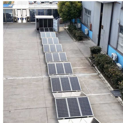
Sao Tome Photovoltaic Energy Storage Power Station
