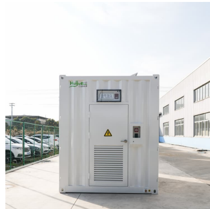
Capacitor energy storage control cabinet
