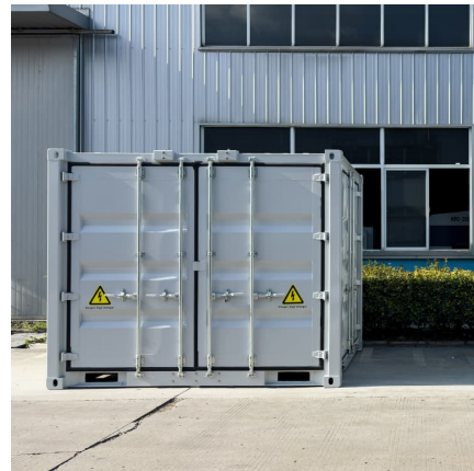
Container energy storage device in ouagadougou
