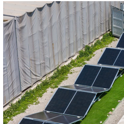
New energy storage configuration in Luxembourg city
