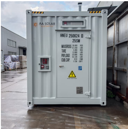
luxembourg city energy storage power station revenue
