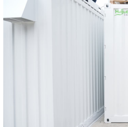
Luxembourg city air energy storage power station
