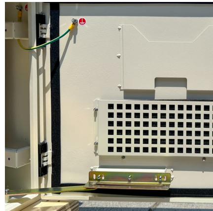
Malabo fengqiao energy storage power station
