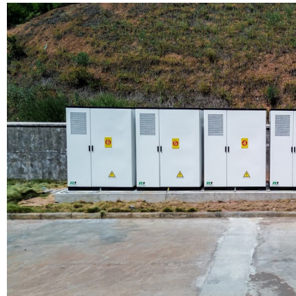
Battery energy storage system (BESS) container. ...
