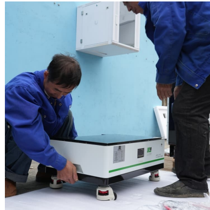
Gitega transfer station equipment energy storage group
