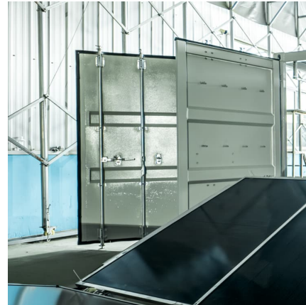
Energy storage battery cabinet disassembly pictures
