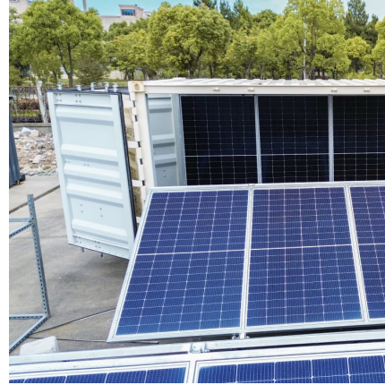
Containerized energy storage , Microgreen.ca
