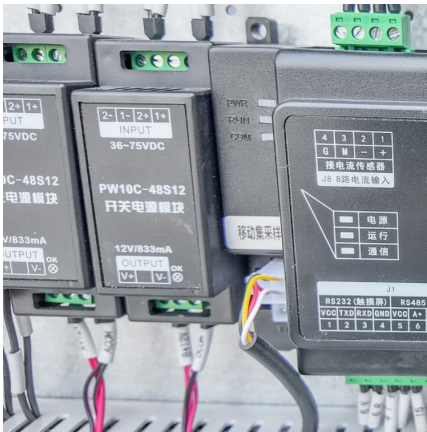
Botswana power grid energy storage station
