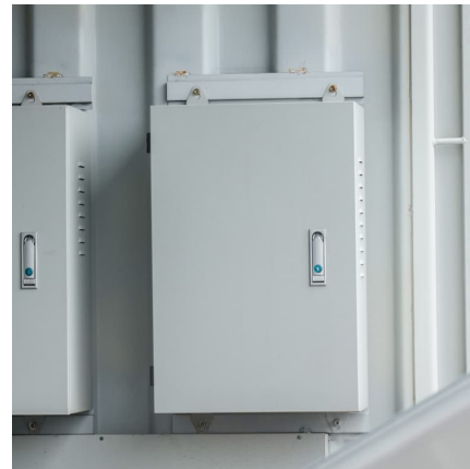
Battery energy storage power station in botswana
