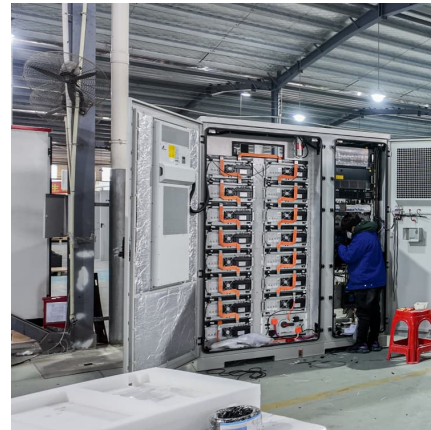
Updated May 2020 Battery Energy Storage Overview
