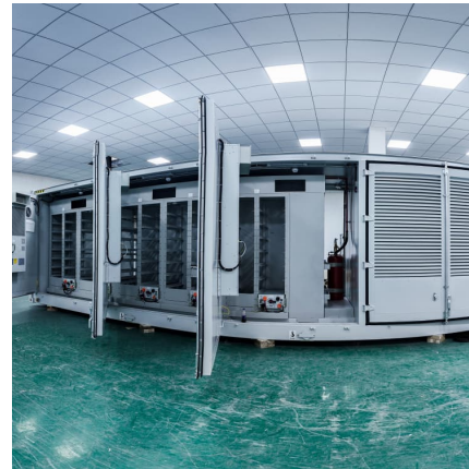
Commercial Battery Storage , Electricity , 2023 , ATB
