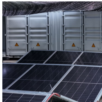
Hybrid power plants, solar+storage were big in 2022, ...
