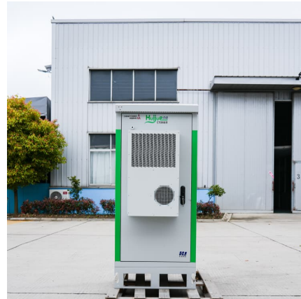
Containerized energy storage , Microgreen.ca
