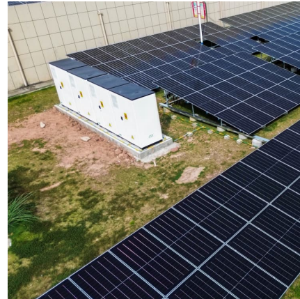
BESS-BYD ground stack Module 100KWh 85KWh 70KWh...
